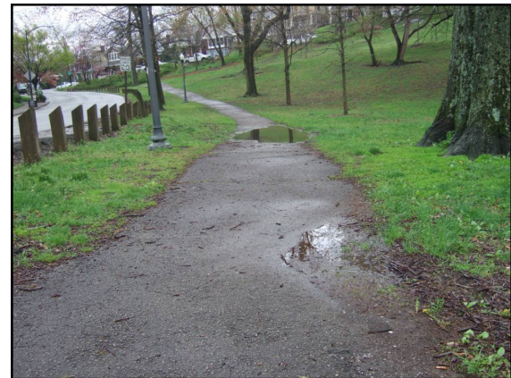
24. Sidewalk into park along Tyler Park Drive, standing water near lightpole
