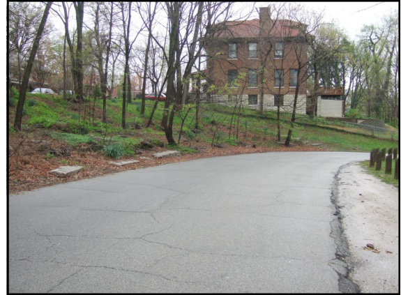
2. View of Tyler Park Drive from Baxter Ave., looking northeast, alligator cracks, shoulder raveling at gravel parking area
