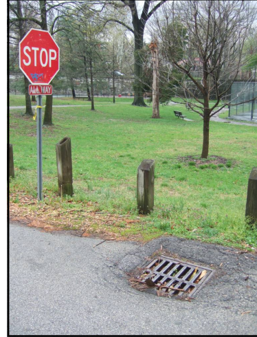
14. Catch basin near the intersection of Tyler Park Drive and Tyler Parkway
