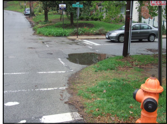
22. Standing water at intersection of Tyler Park Drive and Tyler Parkway
