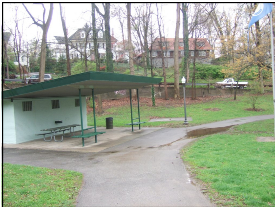
41. Standing water on sidewalk in front of bathroom
