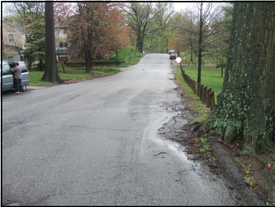
9. Asphalt cracks near large tree along Tyler Park Drive
