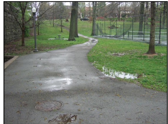
36. Standing water near edge of pavement at east end of tunnel
