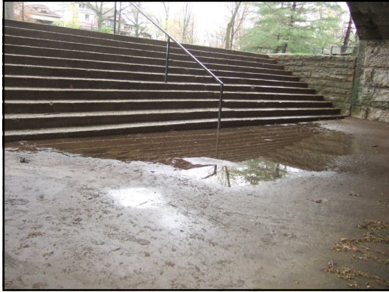
37. Standing water at base of stairs, east entrance to tunnel
