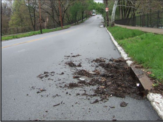
67. Debris and leaves cleared from curb inlet along northeast side of Baxter Ave.
