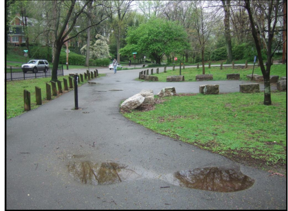
50. Puddles near west entrance
