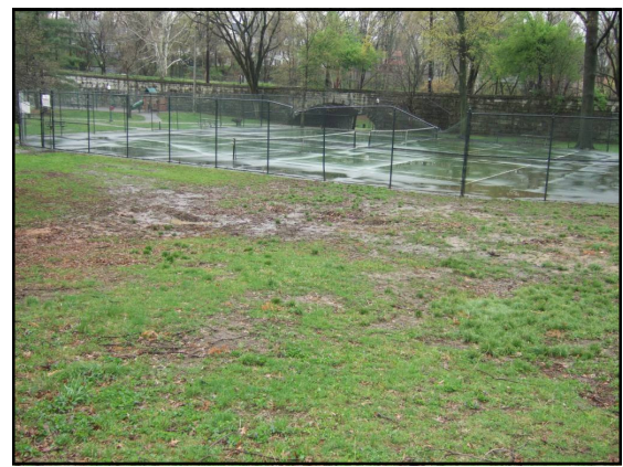
12. View of poor drainage east of north tennis courts
