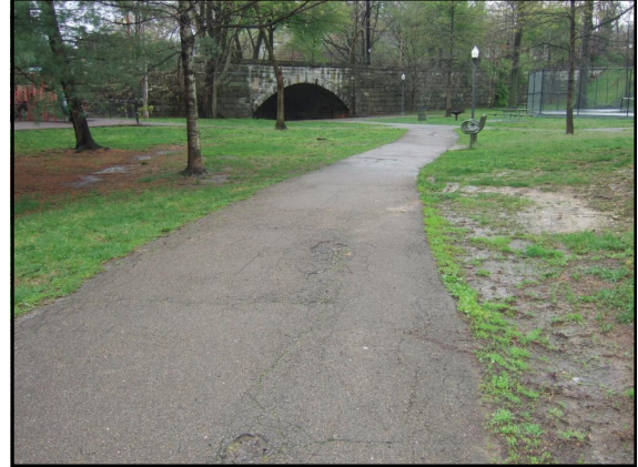
32. Sidewalk leading to tunnel beneath Baxter Ave, minor cracking, poor drainage to the northeast
