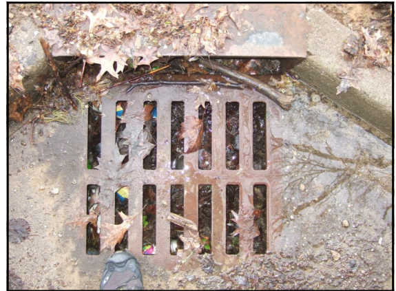
40. Leaves and debris clogging catch basin
