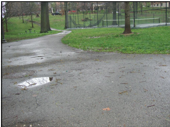
35. Small puddle near east entrance to tunnel
