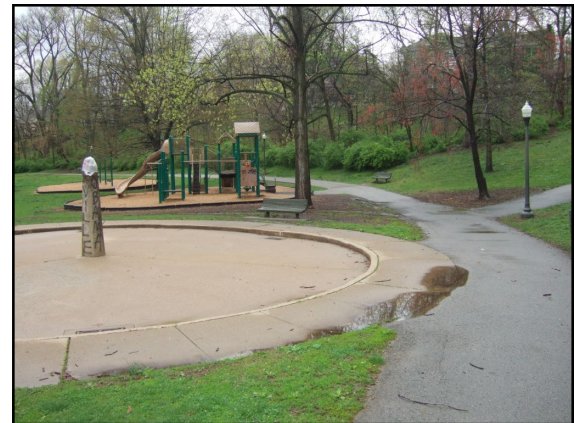
42. Standing water along east edge of spray fountain
