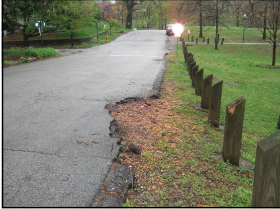
13. Missing asphalt section along the west edge of Tyler Park Drive
