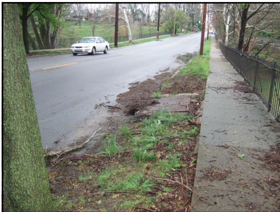
59. Curb inlet along southwest side of Baxter Ave, clogged with leaves
