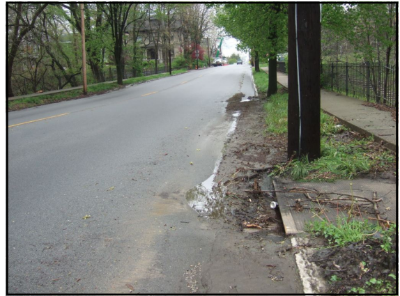
70. Poor roadside drainage, partially clogged curb inlet along northeast side of Baxter Ave.
