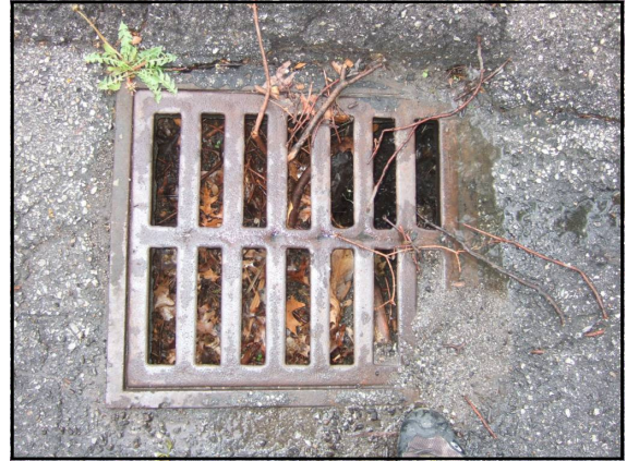
10. Catch basin clogged with leaves
