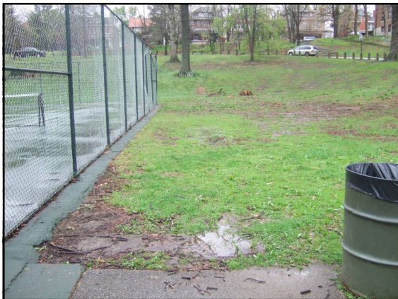
17. Standing water adjacent to north tennis courts
