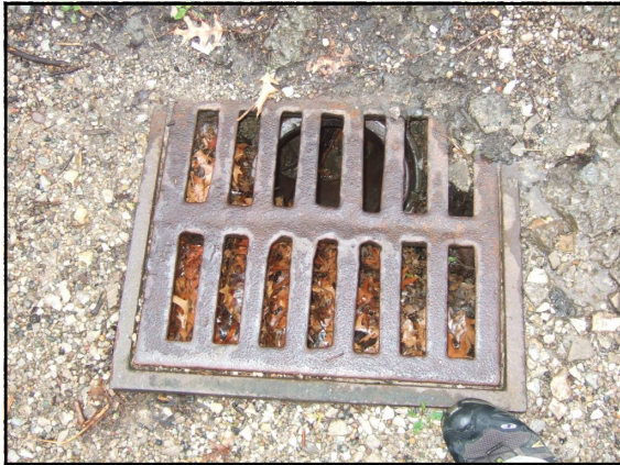
21. Leaves clogging catch basin, with outlet pipe primarily clear
