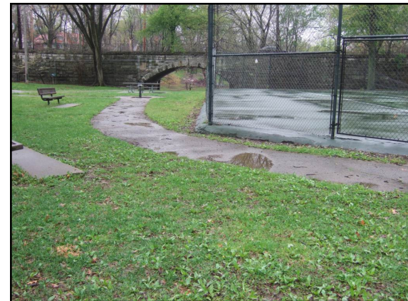
18. Standing water on sidewalk east of north tennis courts
