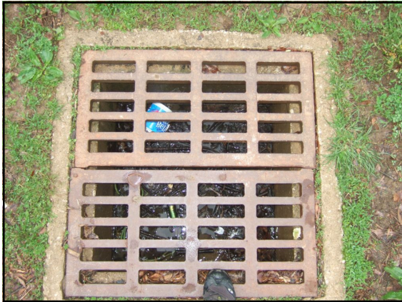
45. Catch basin south of spray fountain, leaves and debris floating
