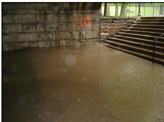
73. Standing water at base of stairs on east side of tunnel
