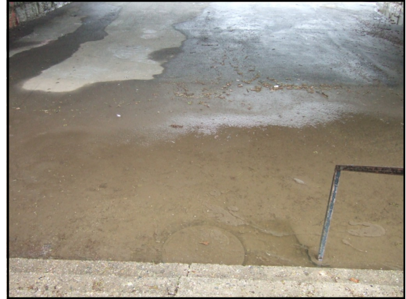
38. Standing water at base of stairs, manhole submerged
