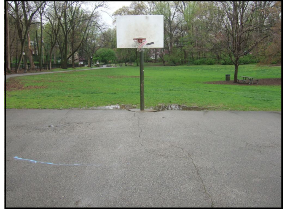
46. Poor drainage behind basketball goal
