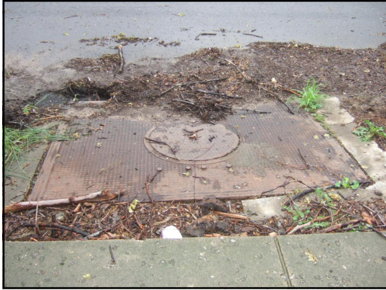
61. Clogged curb inlet along Baxter Ave.
