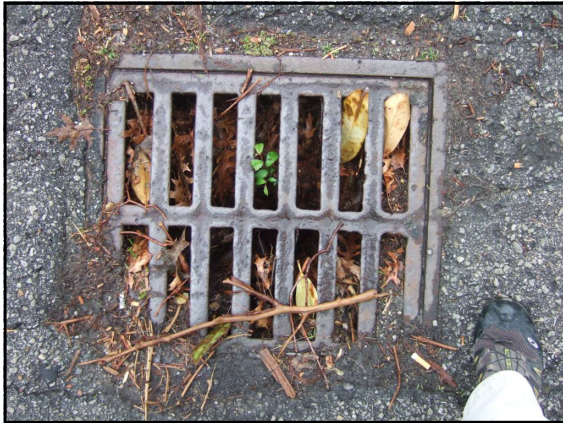
15. Catch basin clogged with leaves
