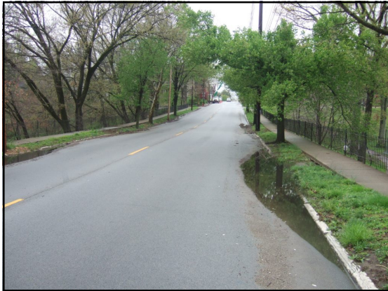
63. Standing water along northeast side of Baxter Ave.
