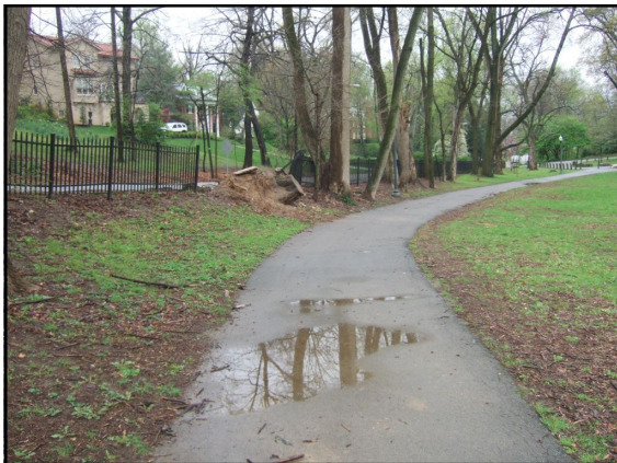
47. Standing water on sidewalk near Castlewood Ave.
