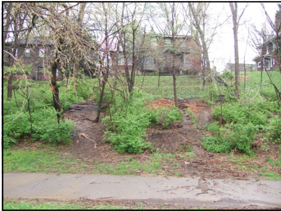
51. Erosion on slope north of west side of park, runoff coming from Tyler Park Drive
