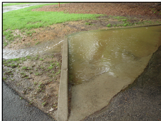
74. Standing water at catch basin, west entrance of tunnel
